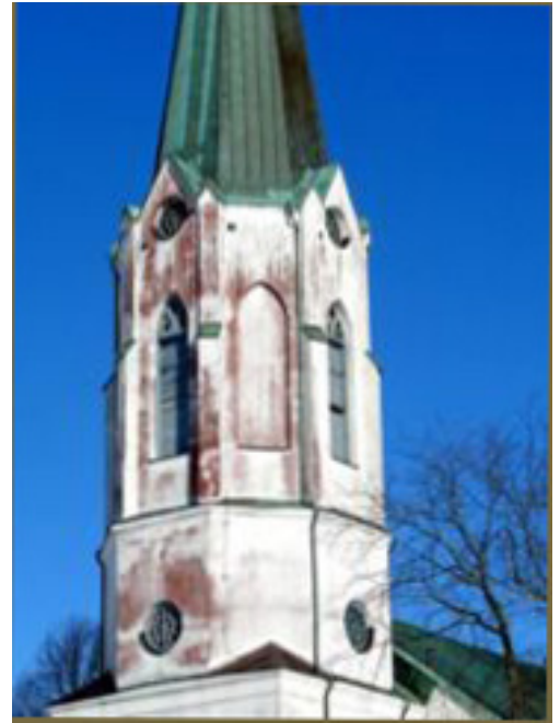
The tower as it looked before the renovation started. The red color is red algae that has arisen in connection with moisture damage.
